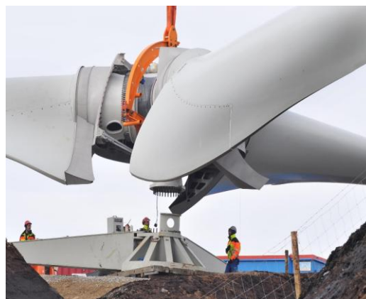
Construction at the new 10MW Caherdowney wind farm operated by Energia Renewables
